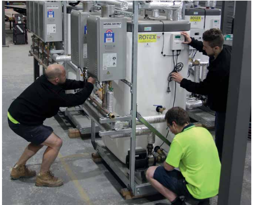
Licensed plumbers are employed to assemble and build the plant packages that are shipped to job sites all over the country.
